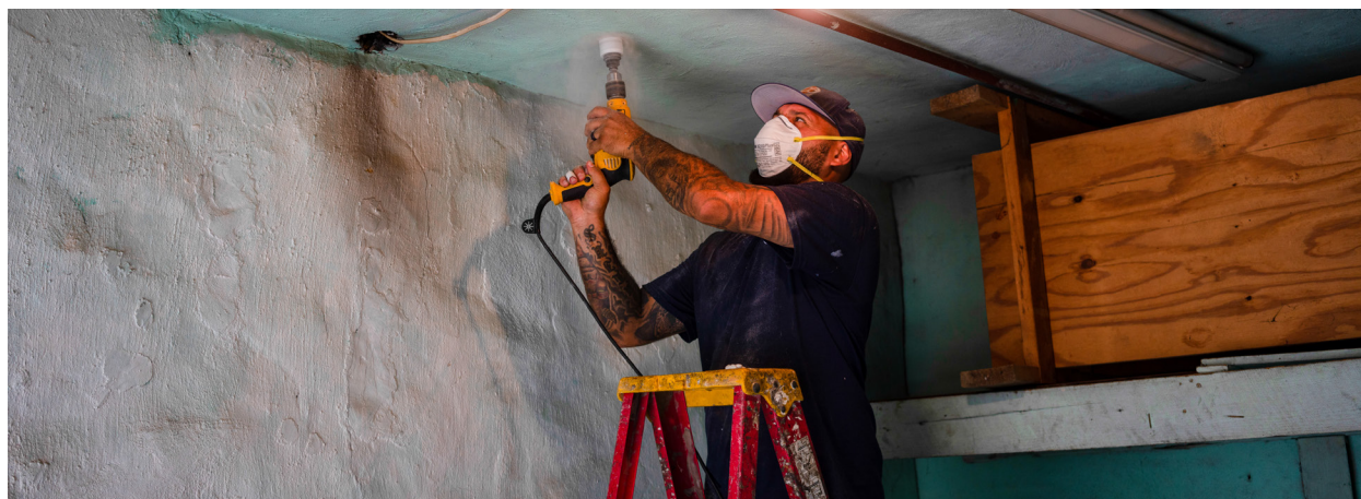
A trainee with the Energy Coordinating Agency performs work to improve the energy efficiency of a Philadelphia home.
