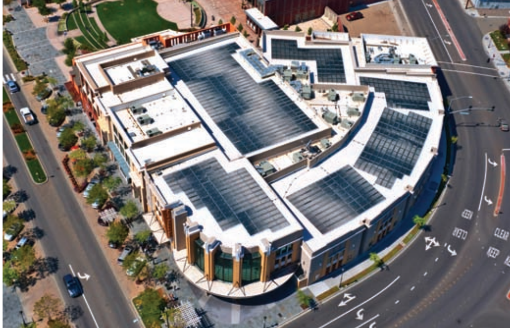
The roof of Cinema West’s Livermore (Calif.) Cinemas, which has a solar-power system from Solyndra Inc., a manufacturer of photovoltaic systems designed to optimize solar electricity production on commercial rooftops. Courtesy of Solyndra.
