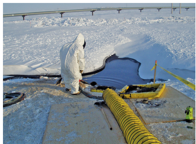
March 3, 2006: Cleanup of GC-2 oil spill that released 212,000 gallons of crude oil in the largest spill on the North Slope. Oil spilled from a quarter-inch hole in the pipeline, caused by corrosion. Nearly two acres of tundra and frozen lakes were impacted.
