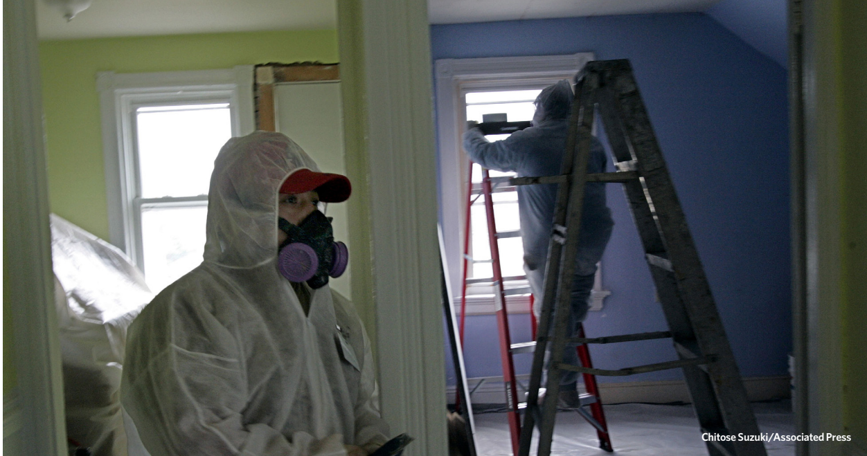
Luis Benitez (left) and Jose Diaz remove lead paint in a contaminated building in Providence, Rhode Island, in 2006.
