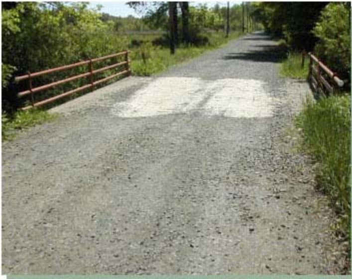
An existing road and bridge in the Great Swamp National Wildlife Refuge similar to the old Meyersville Road, May 2002
