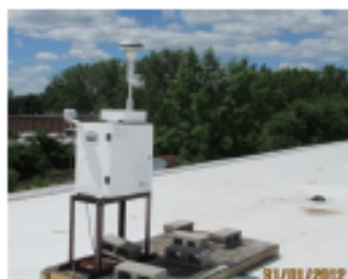
Air monitor on roof of school
