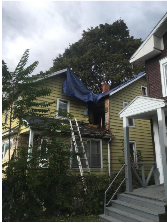
Figure 1 Example of substandard housing.
