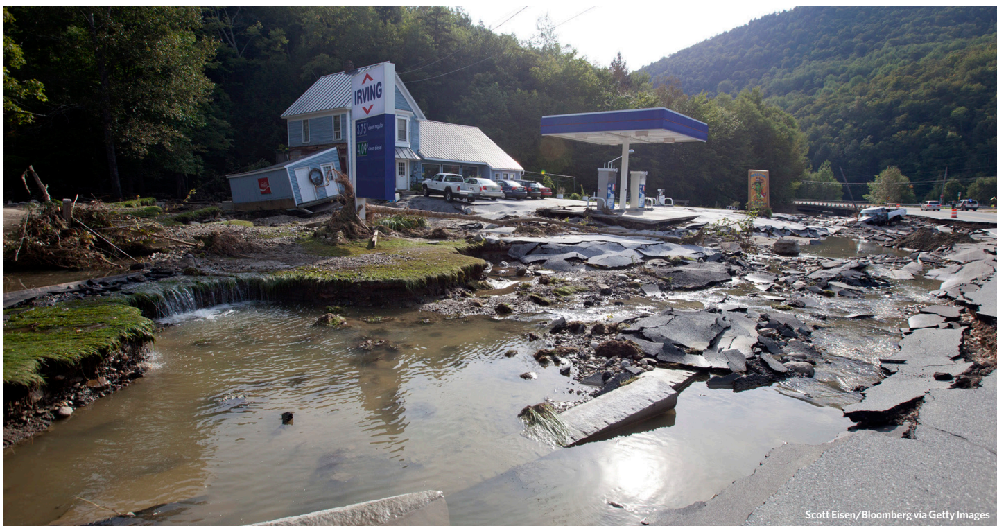
Severe floods from Tropical Storm Irene tear up the asphalt and damage a building at a gas station at the junction of routes 4 and 100 in Killington, Vermont, on Aug. 31, 2011.
