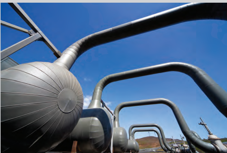
Geothermal power station in Iceland.
