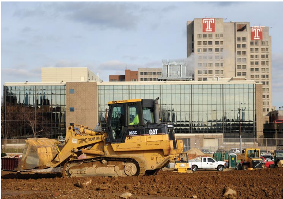
The John Wanamaker School in North Philadelphia has been demolished to make way for a 14-story, 238-unit apartment tower with ground-floor retail and parking. The project will house Temple University students.
