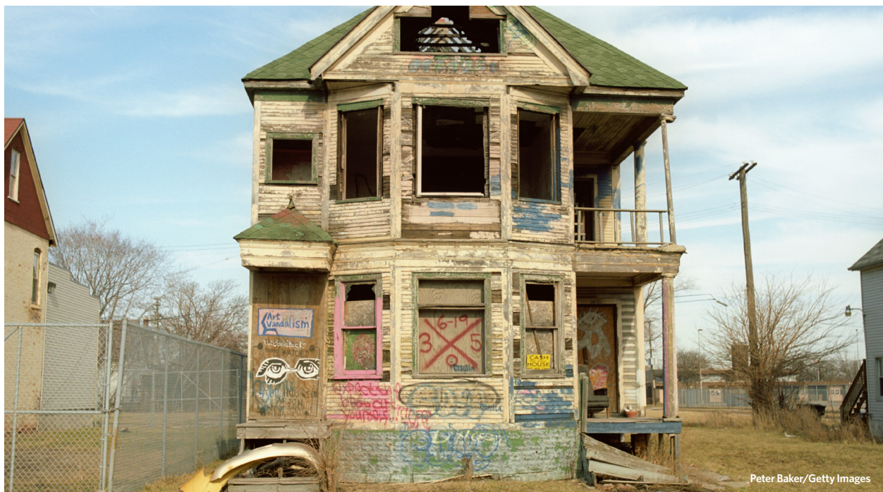
Graffiti covers an abandoned house in Detroit. The city’s initiative to track blight helped a task force recommend which neighborhoods should receive property remediation funding.
